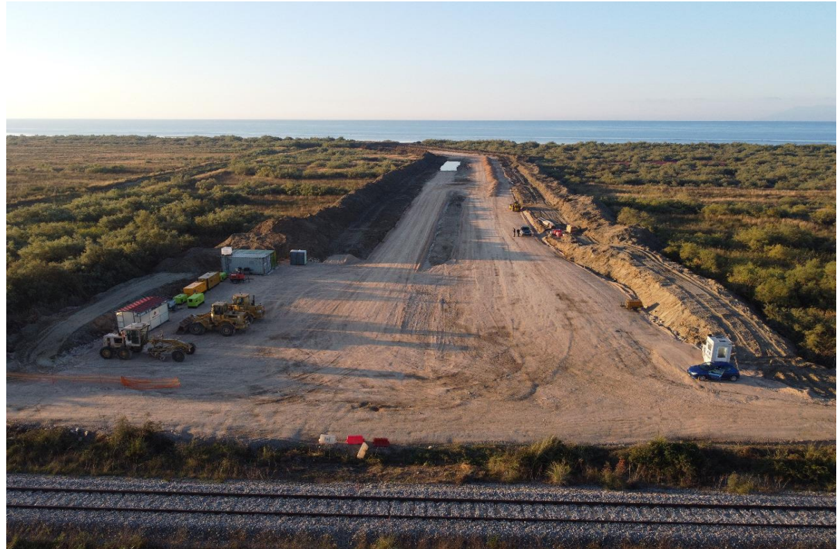
Onshore Right of Way Construction Works from the railway to the shoreline completed (390 m)
